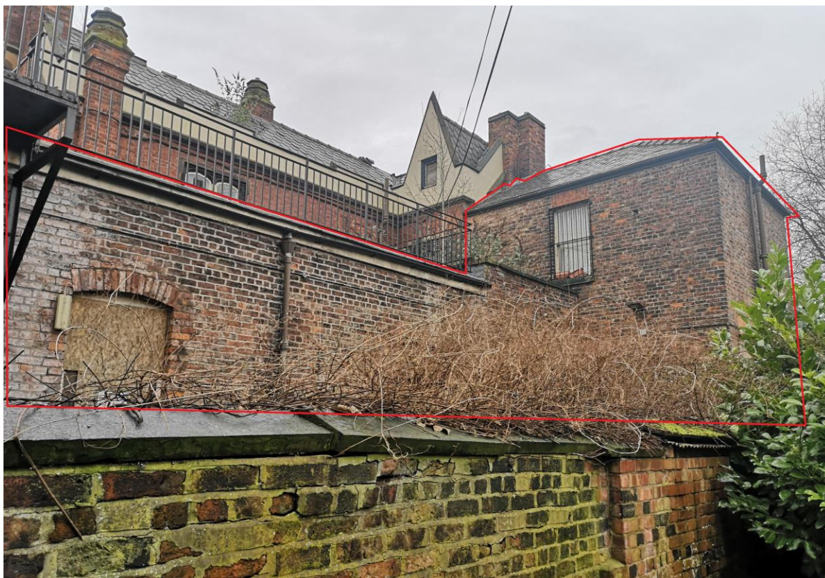
Photograph of the rear of High Elms with later extensions edged red
